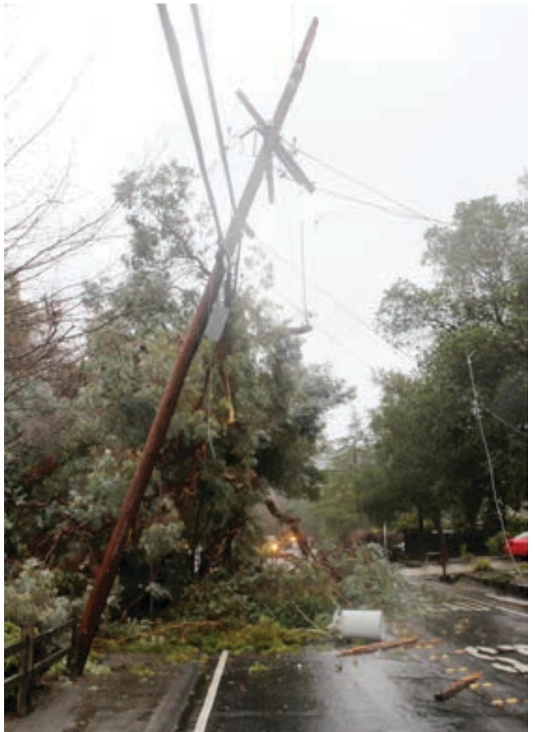
Many power lines are in danger to be damaged by falling trees like this one on Reliez Valley Road.
